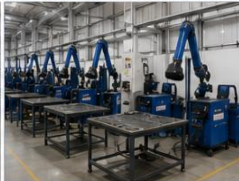
5 WELDING & FABRICATION AREA (TIG / MIG / SPOT)
